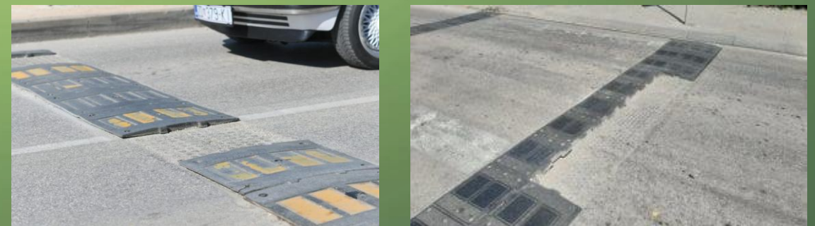
Damaged rubber elements
